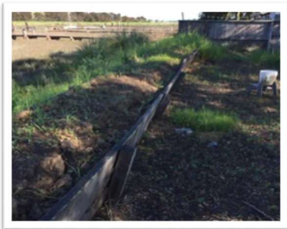
Above: An example TRB that needed to be rebuilt.
