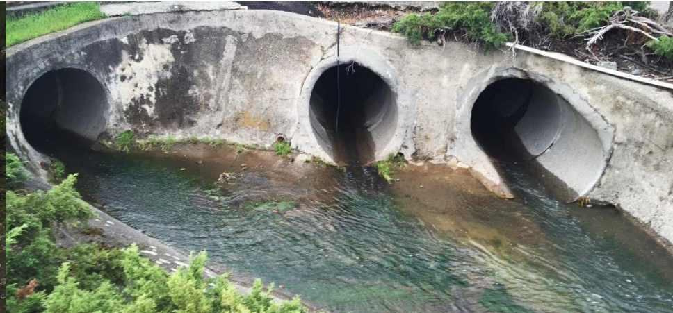
Poor water quality
