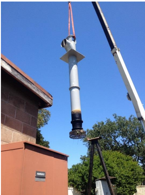
Station #3 pump before service
