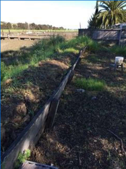
Timber Reinforced Berm in need of repairs
