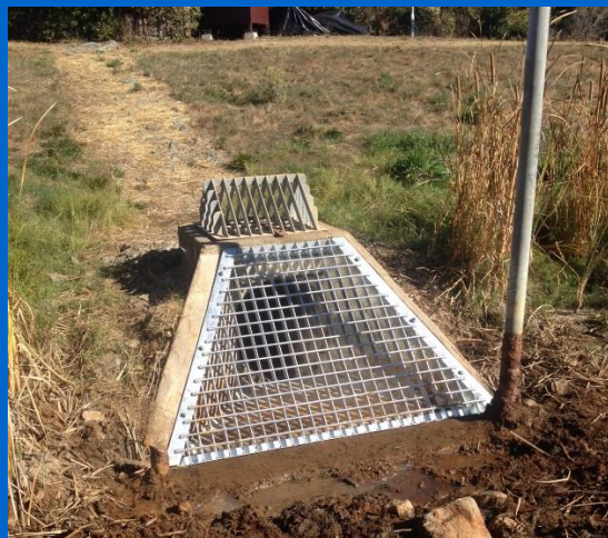
New trash rack at Pump Station 4 inlet
