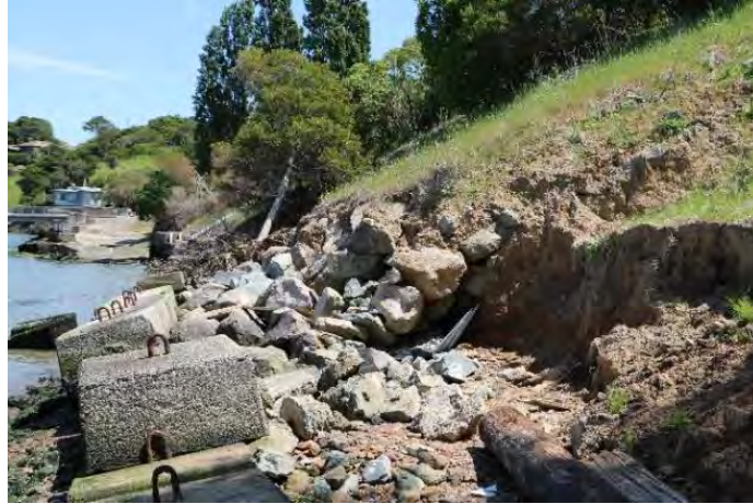
Figure 5: Concrete blocks and riprap failing to protect the slumping bluff at Paradise Beach Park. Note the tree is lying at an angle due to the slumping of the slope. This photo was taken at high tide, and the beach is very narrow, providing no recreation value or protection to the bluff from breaking waves.
