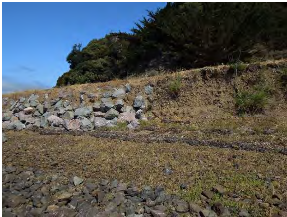
Figure 6: Riprap used to protect the slumping bay cliff along Seminary Drive.
