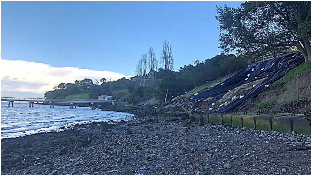
Figure 39: Concrete blocks and riprap failing to protect the slumping bluff. This photo was taken at mean tide and you can see that the beach is not accessible for recreation and does not provide any protection to the bank from breaking waves at tidal levels above mean tide. The result is wave attack to the toe of the backshore bluff occurs through much of the tidal cycle whereas Seminary and Greenwood beach in Richardson Bay only see wave action at tidal levels above +2 ft and +3 ft, respectively.
