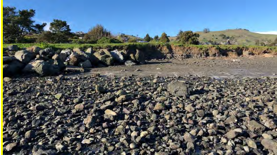
Figure 4: Eroded bank and boulder riprap at Greenwood beach. The coarse cobble-size material in the foreground is composed of asphalt and concrete rubble that waves erode from the lower layer seen in the steep bank. Once eroded from the bank, waves can move this material across the mudflat, providing evidence for the level of wave competence active at this site.
