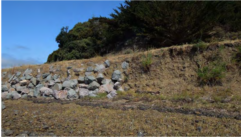
Figure 74: Riprap used to protect the slumping bay cliff that forms the edge of Seminary Drive and the eroding vertical bank that is not protected and exposed to wave action during high tides.
