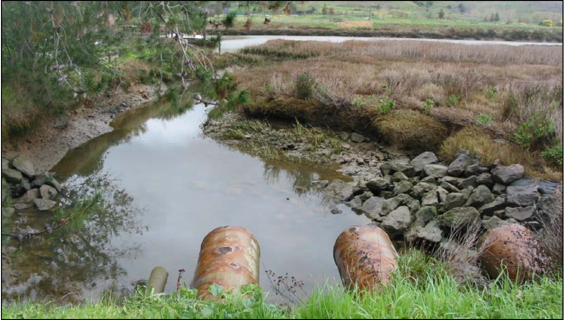
Figure 7. Outlets at Pump Station No. 5
