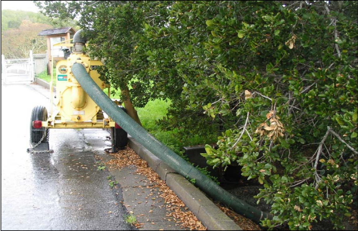
Figure 4. Portable Pump Located at Meadow Drive
