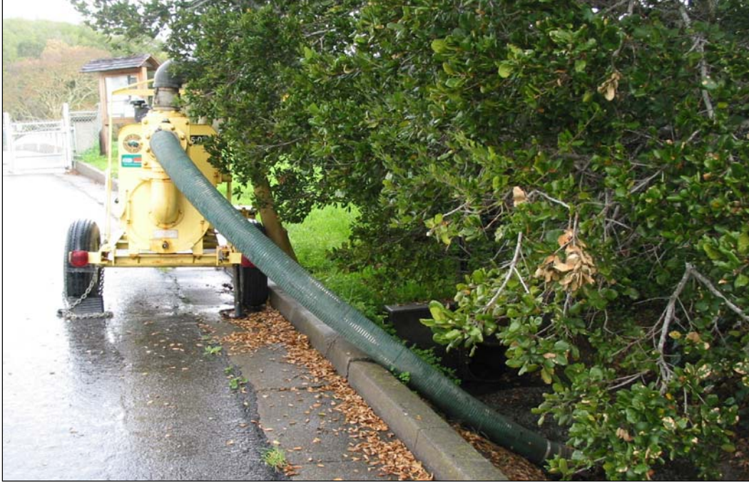
Figure 2.1. Portable Pump Located at Meadow Drive
