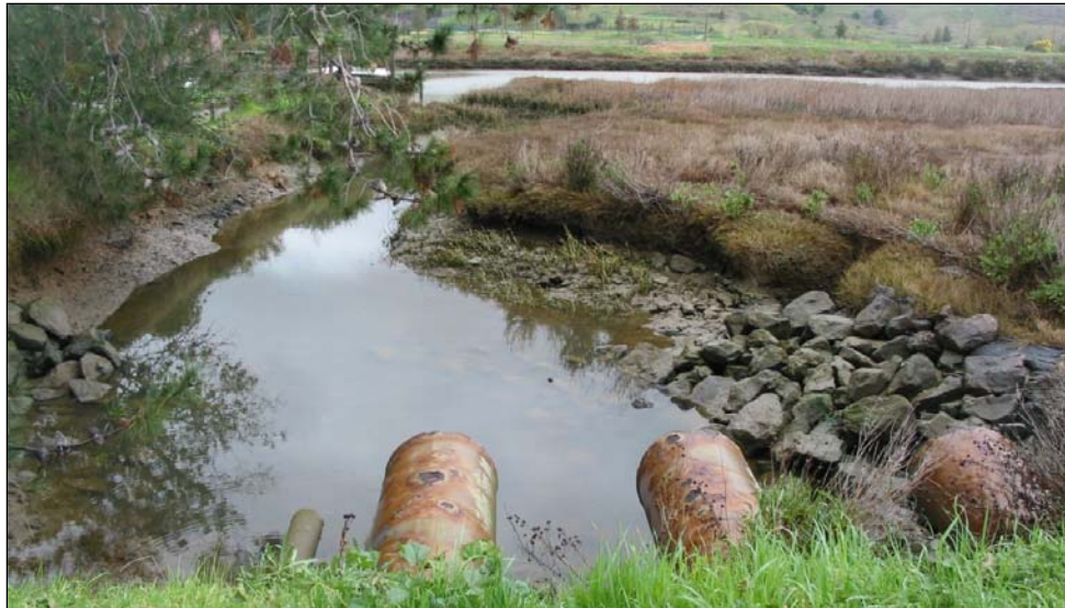
Figure 2.4. Outlets at Pump Station No. 5
