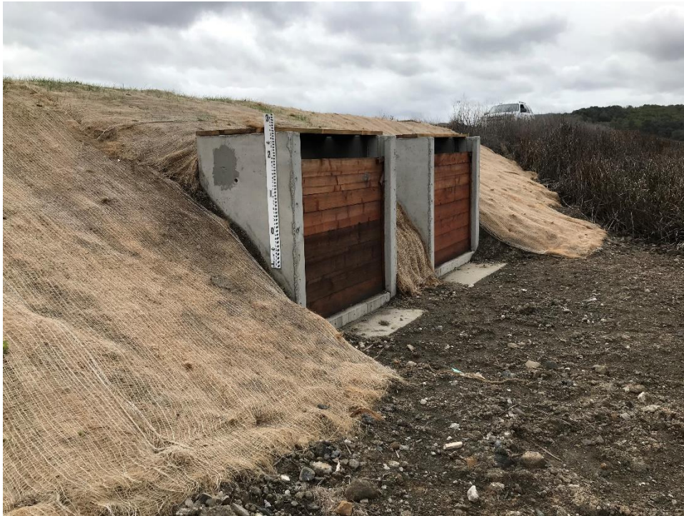
New water control structures to enhance seasonal wetlands at the Audubon property
