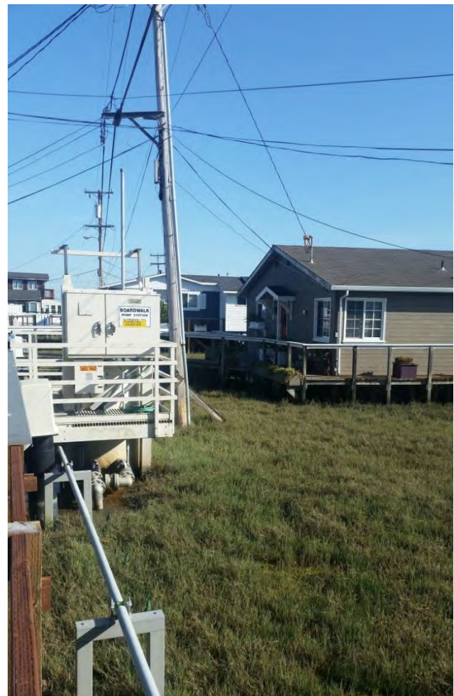
Greenbrae Boardwalk utility lines and control systems. Credit: BVB Consulting LLC
