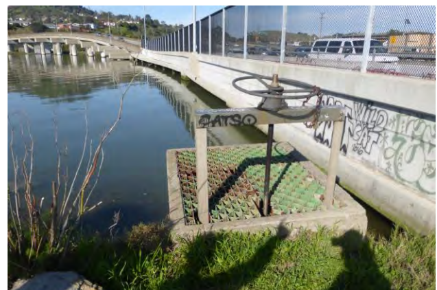
Corte Madera Creek at the end of Lucky Drive. Note the low-lying segment of US Highway 101 starts here. Credit. Marin County DPW
