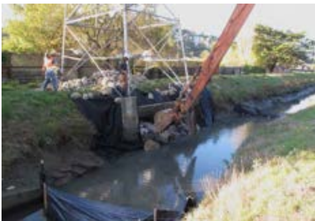
PG&E repair from storm damage in Tamalpais Valley. Credit Marin County DPW
