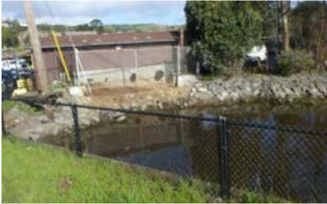
Pump station and overflow pond at the Cove Shopping Center. Credit: Marin County DPW
