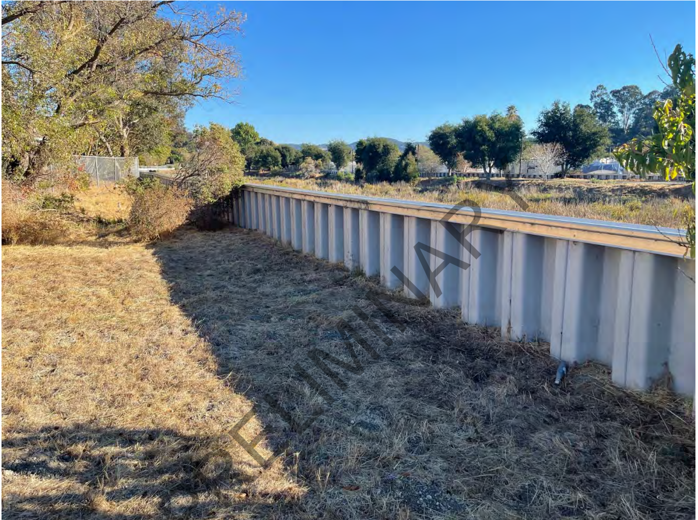
Figure 18 Composite Sheet Pile located along Pinole Creek in Pinole, California
