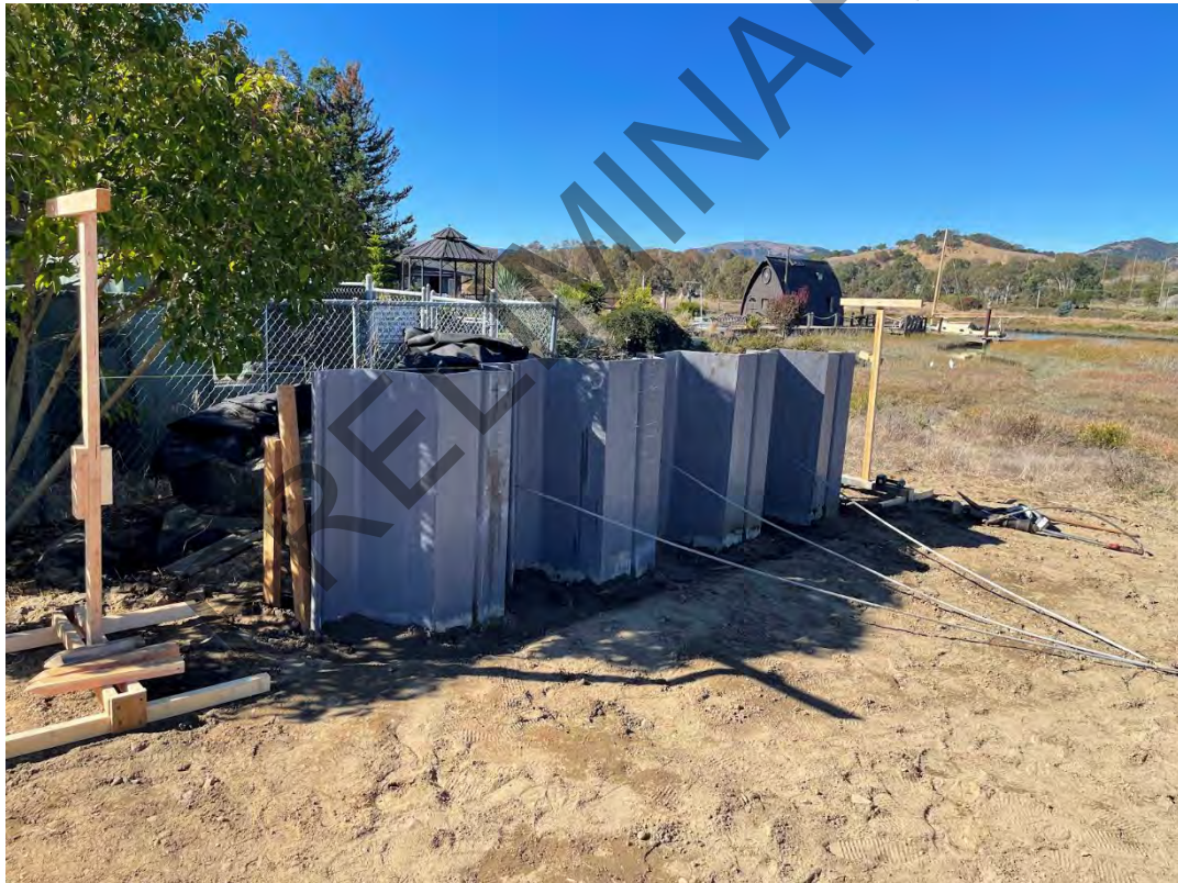
Field test of floodwall near Pump Station Number 5. See Appendix C for details.
