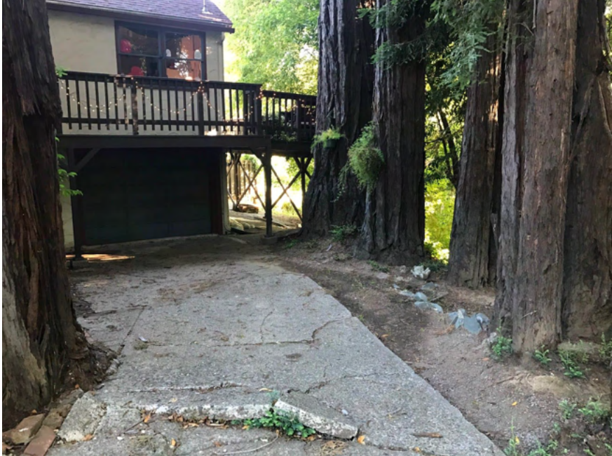
View of lower level adjacent to creek, where flood water enters: garage, laundry room, water heater.
