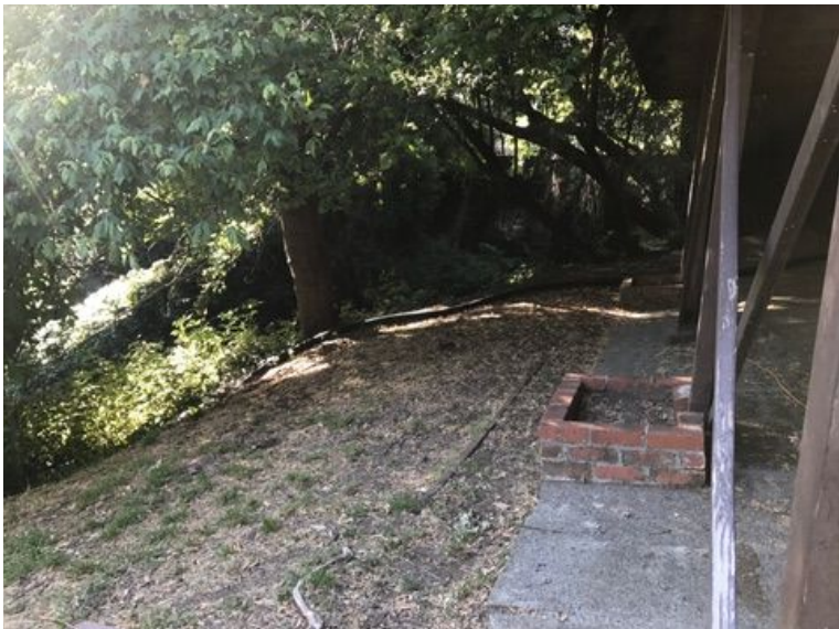
Distance from creek bank to foundation = Where the elevation should be measured.
