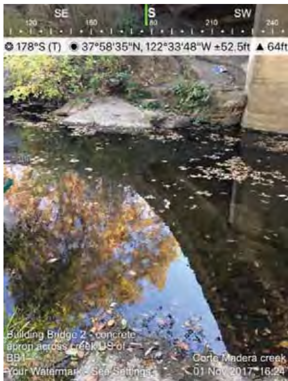
Figure A-16: Concrete Sill Extending across Channel on Downstream Face of Bridge Street Bridge
