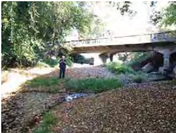
Figure A-8: View of Upstream Face of Nokomis Bridge Notice large gravel bar deposits underneath and in left bay of bridge.
