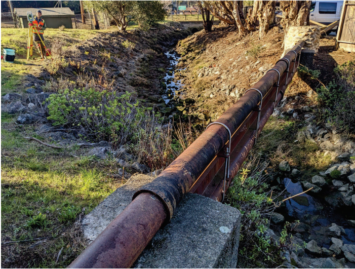
Photo 4. East Creek. Looking from left bank to right bank along the sanitary sewer crossing near Station 1+80' and narrow grouted rock channel with 4.7' invert on the pipeline section (December 16, 2022). See also cover photo.
