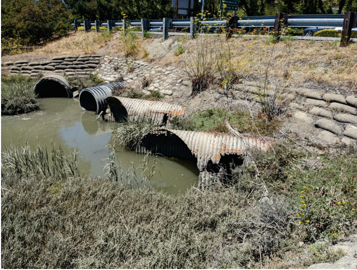
Photo 6. West Creek. Looking from left bank to outlet of two 60" CMP culverts (in foreground) outfalling to open natural channel downstream from Tiburon Boulevard (August 3, 2022).
