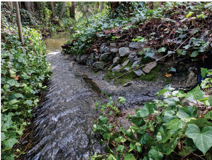
Photo 11. Looking downstream to the grade-controlling channel-spanning concrete stormwater outfall forming a headcut-step on Upper West Creek near Station 11+60' (January 19, 2023).
