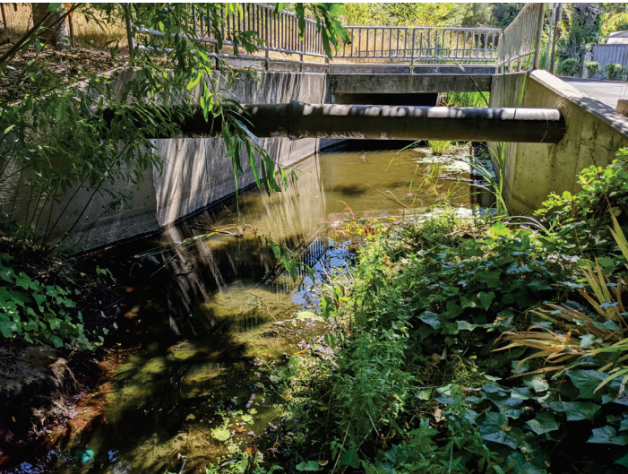
Photo 5. East Creek. Looking downstream from inlet to the 10-ft-wide open concrete box culvert and overhead sanitary sewer pipe crossing to 5'x10' Cecilia Way concrete box culvert downstream in background of view (August 3, 2022).
