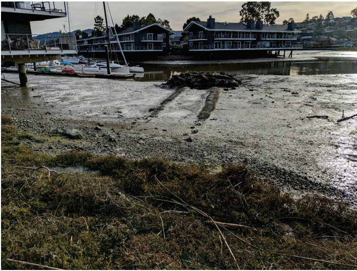
Photo 1. East Creek. Looking downstream to the original double-barrel 60" CMPs outfalling in Richardson Bay near Station -3+95' (January 19, 2023).
