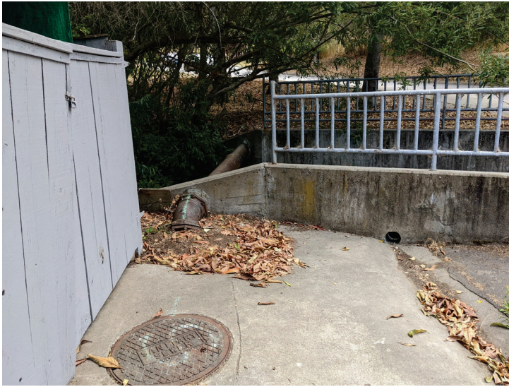
Photo 14. Upper East Creek. Looking from Cecilia Way to the upstream end of the right bank concrete transition channel wall about 30 feet upstream from the Cecilia Way culvert road crossing (August 17, 2022). The stormwater drain hole in the wall discharges creek flow onto the street during routine or average annual high creek flows. Blocking the drain hole combined with surface drainage improvements for directing the concrete swale flows to existing storm drain inlets near the Cecilia-Leland Way intersection should be considered.
