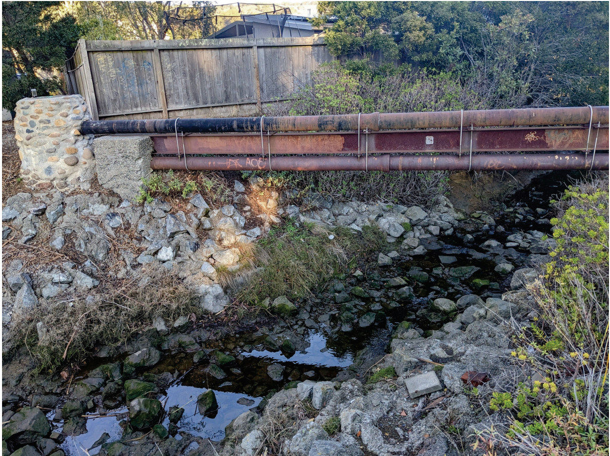
Looking upstream to East Creek from near STA 1+50' to RBSD sanitary sewer pipe crossing (December 16, 2022).
