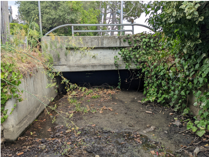
Photo 7. West Creek. Looking upstream to outlet of the Cecilia Way 5.3'x11.4' concrete box culvert (August 17, 2022). Note there is about 2-3 ft of fine sediment deposited within the downstream part of the culvert but much less sediment deposited in the upstream part of the culvert. This is the natural, unmaintained condition.
