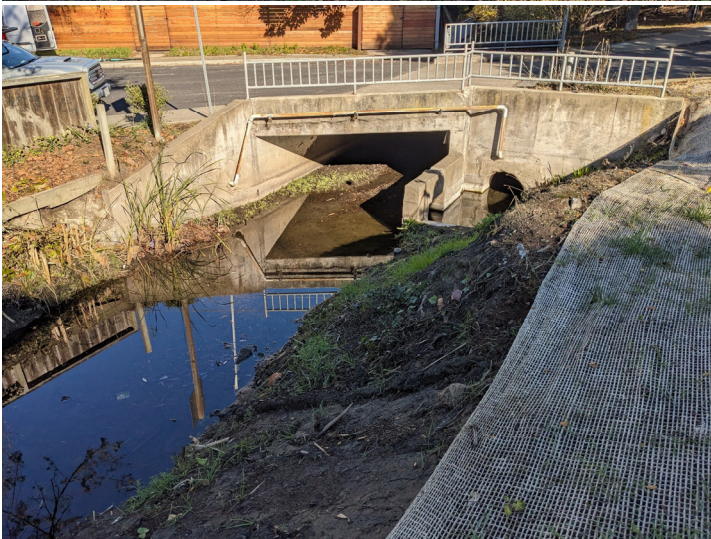
Photo 9. East Creek. Looking upstream to the outlet of Cecilia Way culvert (December 16, 2022). This is the maintained condition following channel maintenance dredging completed in October 2022. None or negligible sedimentation occurred downstream from Cecilia Way culvert during November and December rainstorms.
