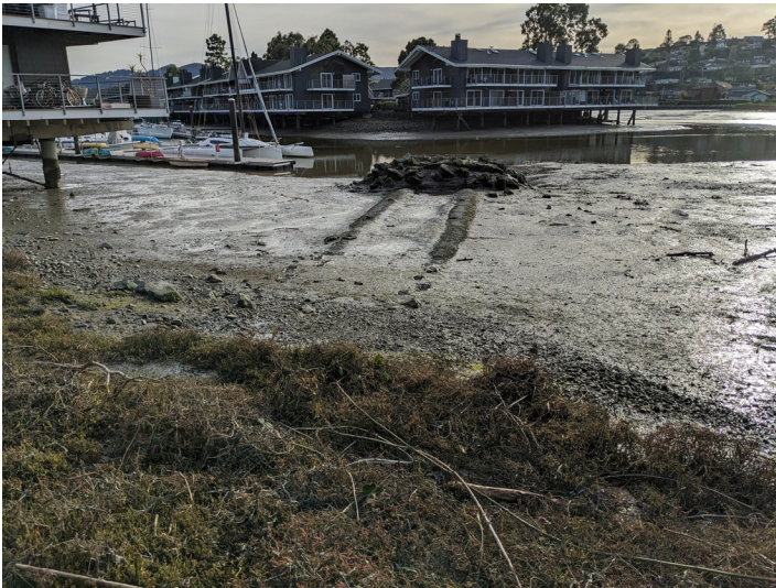
Photo 1. East Creek. Looking downstream to the original double-barrel 60" CMPs outfalling in Richardson Bay near Station -3+95' (January 19, 2023).
