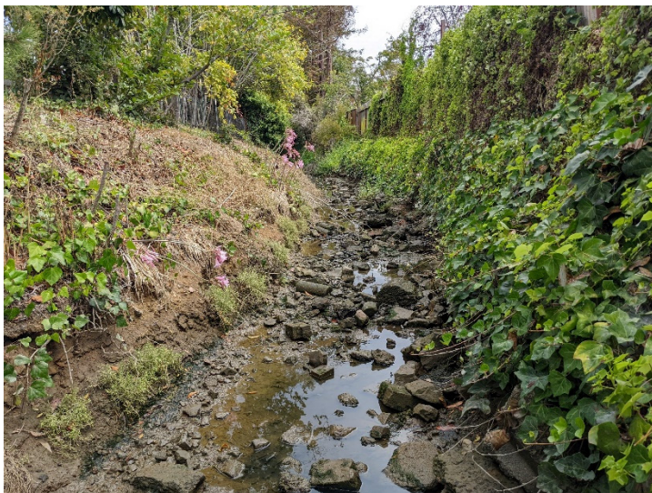
Photo 12. Lower West Creek. Looking upstream from Lower West Creek channel bed near Station 3+00' to the broken concrete rubble covered channel bed (August 17, 2022).
