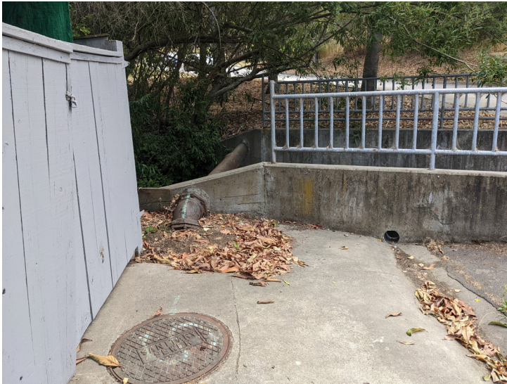
Photo 14. Upper East Creek. Looking from Cecilia Way to the upstream end of the right bank concrete transition channel wall about 30 feet upstream from the Cecilia Way culvert road crossing (August 17, 2022). The stormwater drain hole in the wall discharges creek flow onto the street during routine or average annual high creek flows. Blocking the drain hole combined with surface drainage improvements for directing the concrete swale flows to existing storm drain inlets near the Cecilia-Leland Way intersection should be considered.
