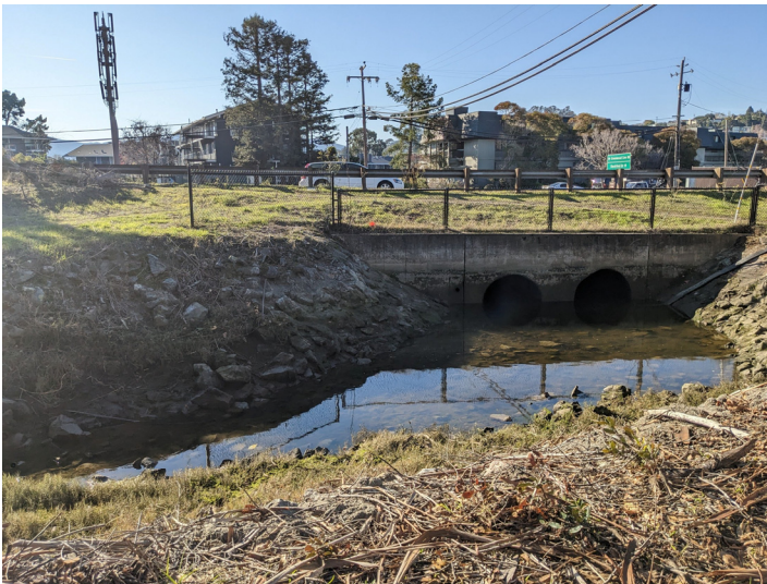
Photo 2. East Creek. Looking downstream from right bank of the grouted rock channel to the vertical concrete headwall inlet to the State Route 131 66" RCP "double-barrel" at Station 0+00' (December 16, 2022).
