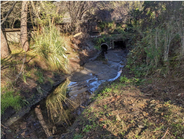
Photo 8. East Creek. Looking upstream to the outlet of culverts originating at or upstream from Karen Way (December 16, 2022). This is the maintained condition following channel maintenance dredging completed in October 2022. Note sedimentation near the culvert outfalls that occurred during November and December rainstorms.
