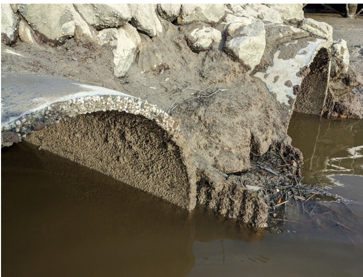
Photo 10. East Creek. View of the East Creek culvert outfalls in Richardson Bay near Station -3+95' (see also Photo 1). The original double-barrel 60" CMPs appear to have been slip-lined with 52" HDPE plastic pipe culverts (January 19, 2023).
