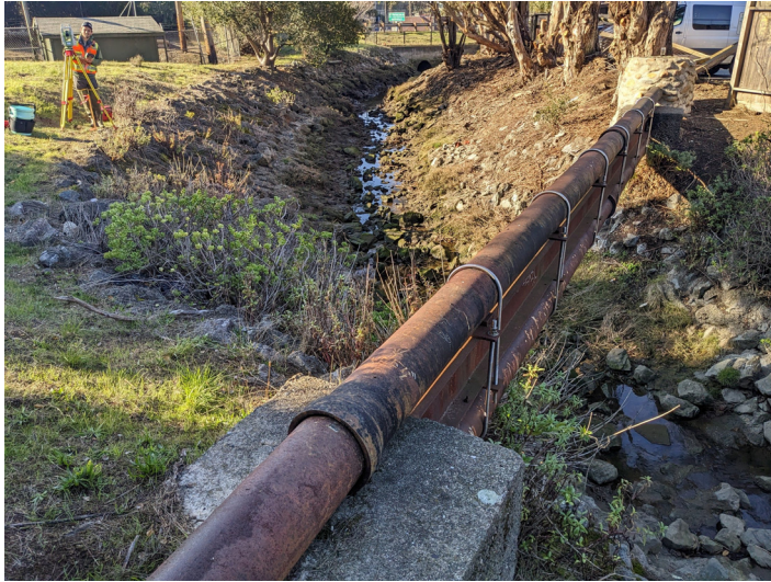
Photo 4. East Creek. Looking from left bank to right bank along the sanitary sewer crossing near Station 1+80' and narrow grouted rock channel with 4.7' invert on the pipeline section (December 16, 2022). See also cover photo.
