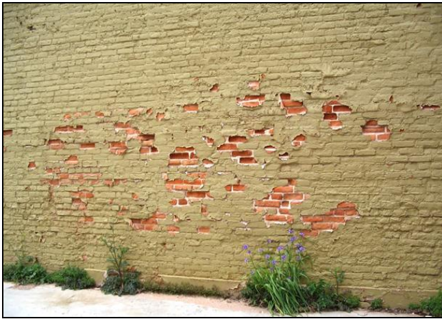
Prepare the surface correctly. Paint has created moisture issues and the surface of the brick has spalled off. Bastrop, TX
