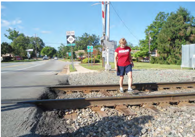
Railroad crossing at Fifth Street lacks a safe place for pedestrians to cross. Pedestrians must either cross the tracks or walk into the roadway.
