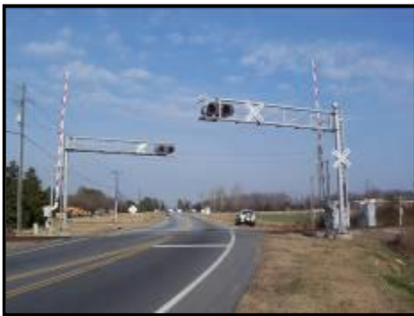
Example of gates, signs and flashing lights
