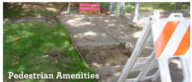
Sidewalk Obstructions and Driveway Ramps
