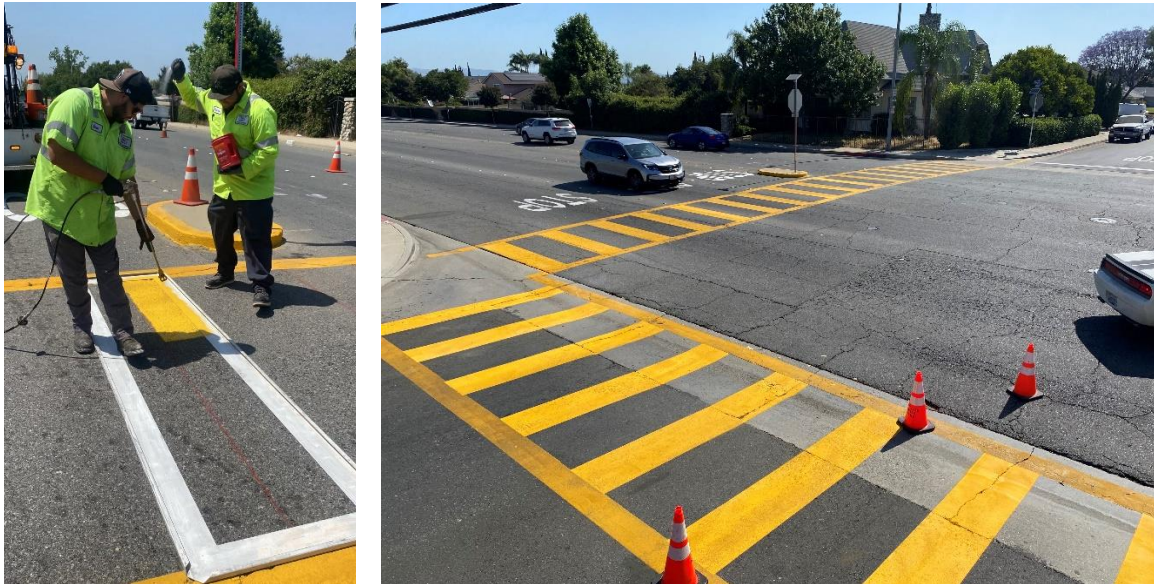
Maintenance workers Aaron Fierro and Nikolas Carbajal striping the intersection of Ramona Avenue and Howard Avenue.
