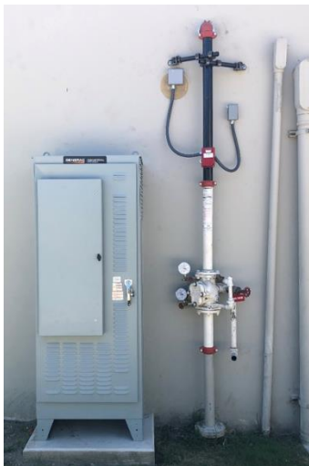
New automatic transfer switch
