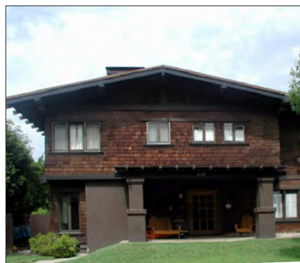
Unpainted siding above painted plaster
