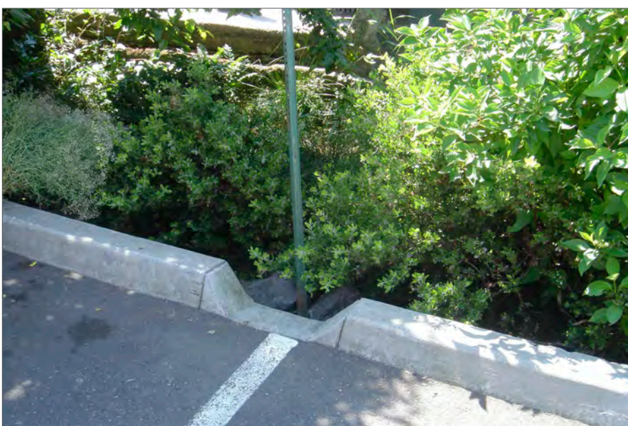
A break in the curb allows water to flow into planters.
