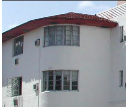
Sloped roofs without gutters
