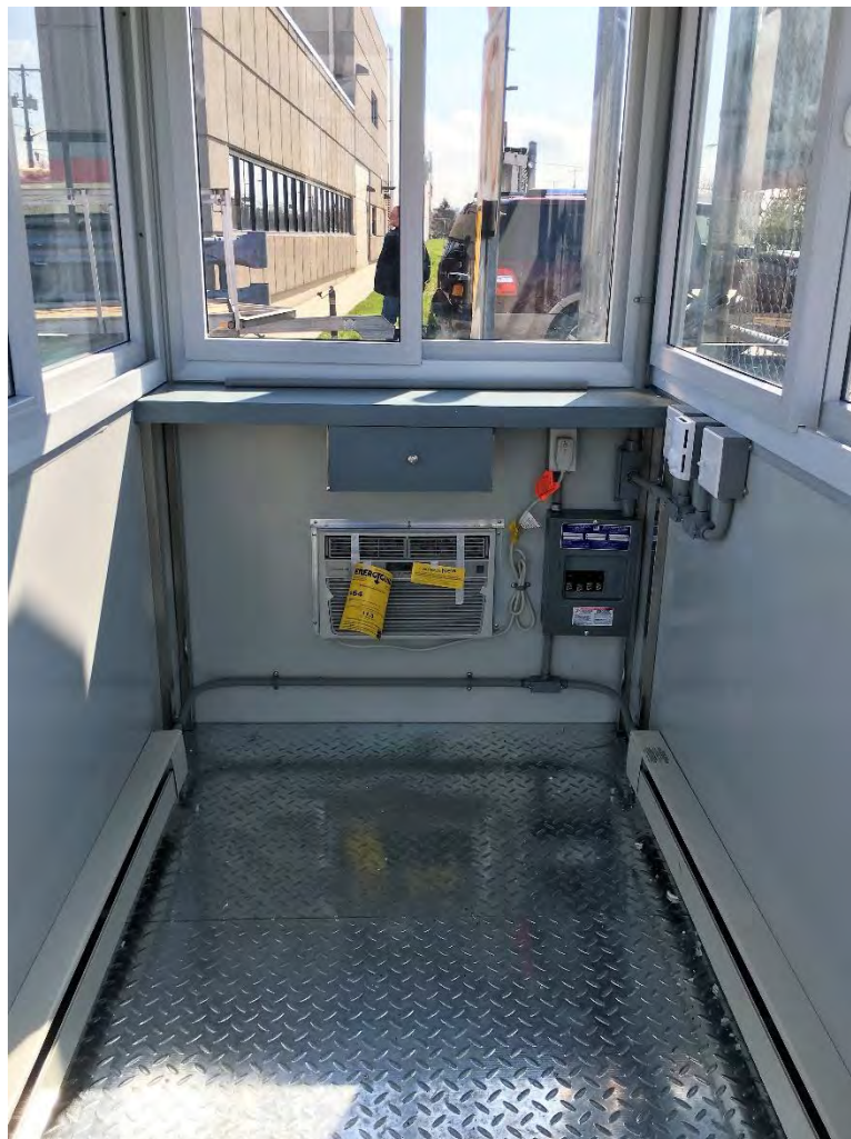
Inside with Heating and A/C units at United Nations
