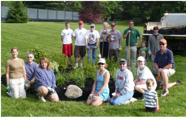
The MCLA class of 2009 volunteered their time and money to install a “raingarden” in Swaim Park.
