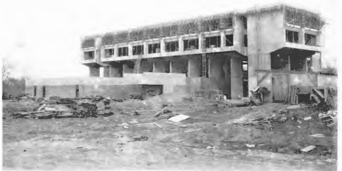
Top photo: former Governor Rhodes at the dedication of the hospital October 15, 1966. Bottom photo shows the progress of the main building construction in 1969.
