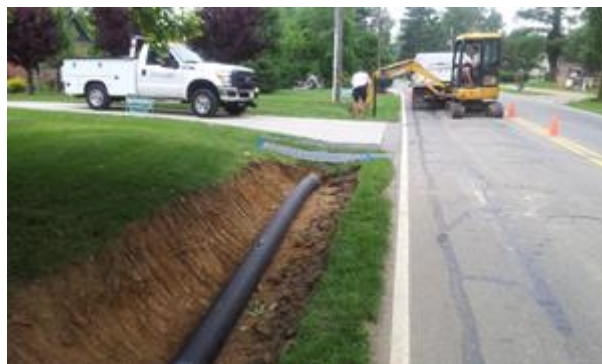
Drainage Improvements in Public Right-of-way
