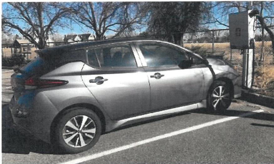
A vehicle-to-building charging station at the North Boulder (Colorado) Community Center is bi-directional, allowing the electric vehicle to feed power to the building at times of peak demand.
