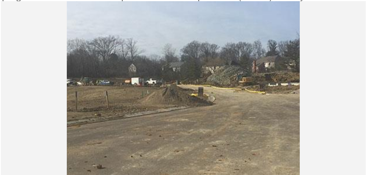
Camden Homes' Orchard Trail subdivision will feature high-end, empty-nester type housing with a pocket park and a walking trail.
