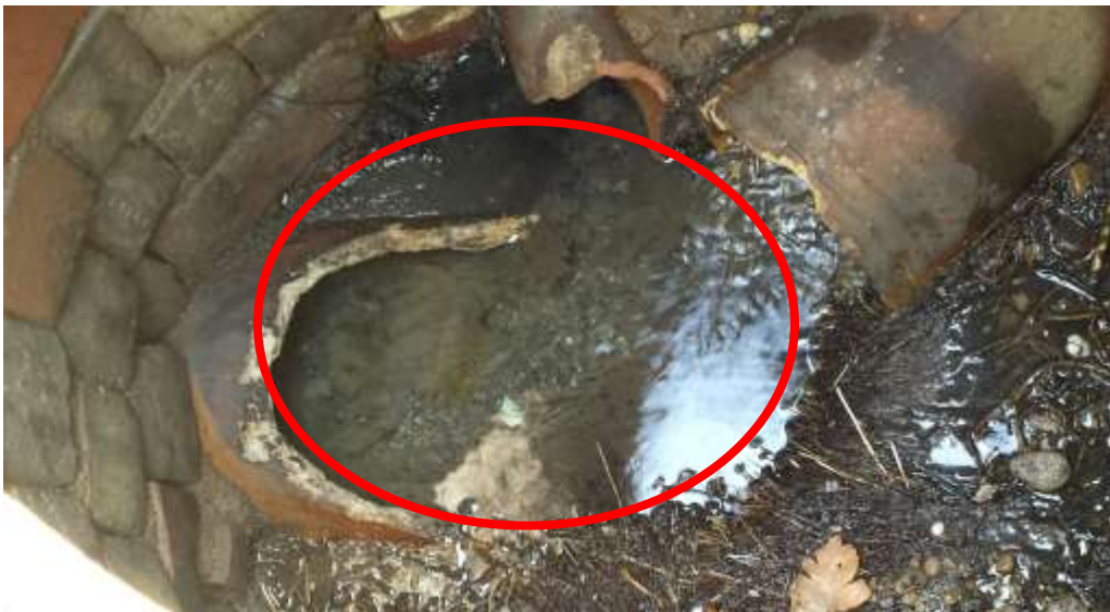
Figure 3: Sewage fungus growing in a stormwater pipe in Moreland
