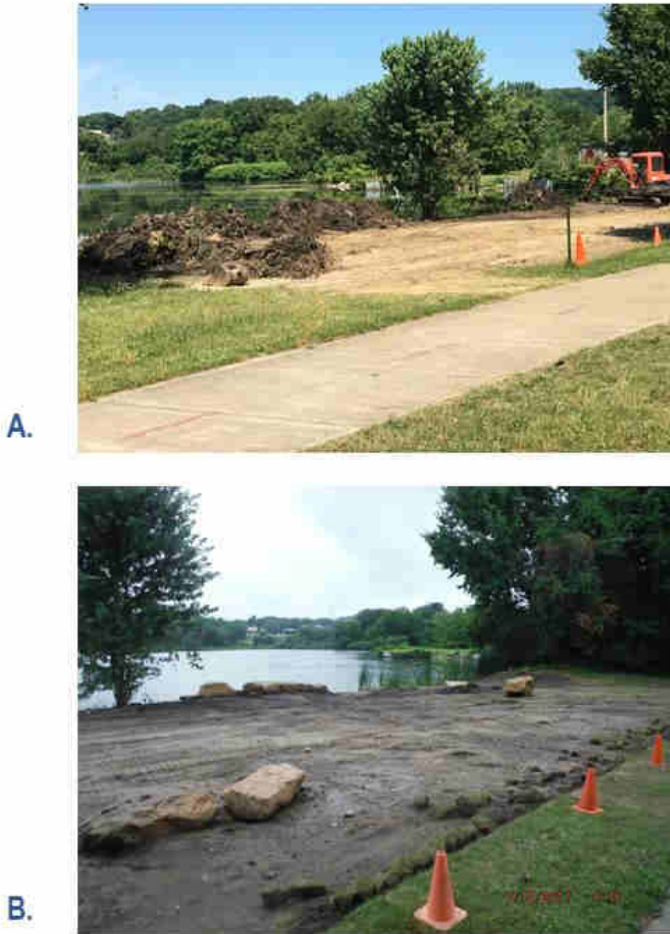
FIGURE 6. SHORE CLEARING AND EARTH MOVING WORK CONDUCTED NEAR THE SUMMIT LAKE COMMUNITY CENTER, JULY 2017: A. JULY 5, 2017; B. JULY 14, 2017.
