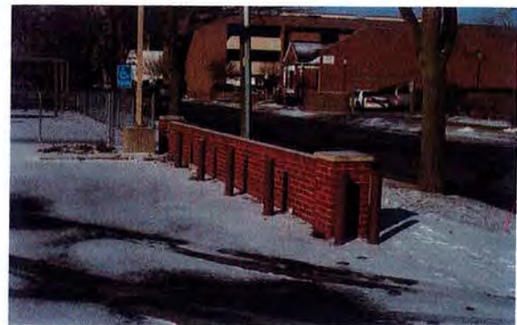
Parking lot with brick screen wall and concrete filled steel bollards to protect perimeter wall
