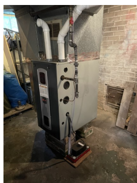
Before and after photos of furnace replaced through a Federal Home Loan Bank grant.
