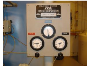
Control Panel at Springhouse
