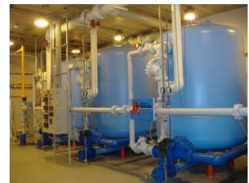
Softening Units at Shafor Water Treatment Plant
