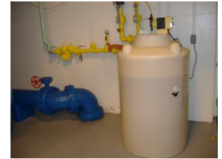
Chlorine Pump at Springhouse
