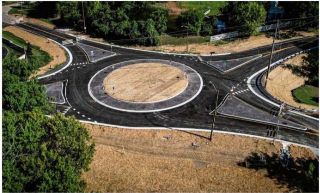
The roundabout at the intersection of Mad River Rd. and West Alex Bell Rd. in Washington Twp. during construction. JIM NOELKER/STAFF
