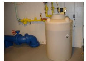
Chlorine Pump at Springhouse
