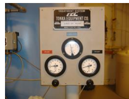
Control Panel at Springhouse
