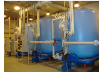
Softening Units at Shafor Water Treatment Plant
