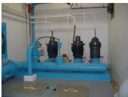
High Service Pumps at Springhouse
