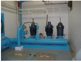
High Service Pumps at Springhouse
