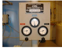
Control Panel at Springhouse
