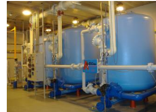
Softening Units at Shafor Water Treatment Plant
