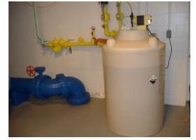
Chlorine Pump at Springhouse
