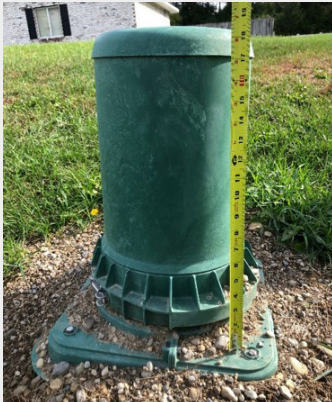
Ground Level Closure Pedestal Size: 18.5 inches tall Number of pedestals in Oakwood: Approximately 200
