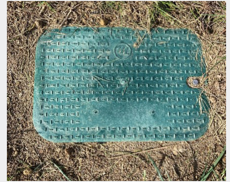
Handhole Fiber Junction Box Size: Flush-mounted and Inground Number of boxes in Oakwood: Approximately 2,000
