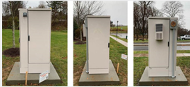
Distribution Hub Cabinet Size: 7 foot tall Number of cabinets in Oakwood: 7
