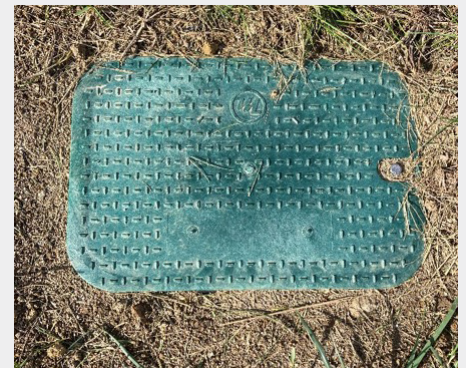
Handhole Fiber Junction Box
