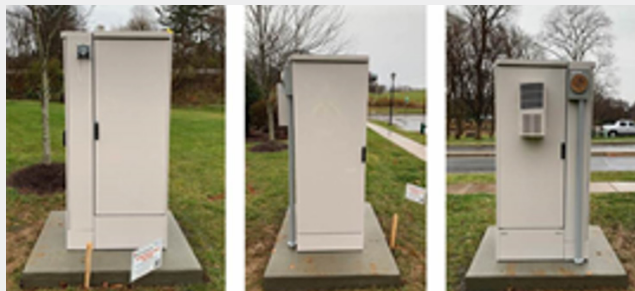
Distribution Hub Cabinet
