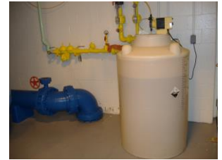
Chlorine Pump at Springhouse
