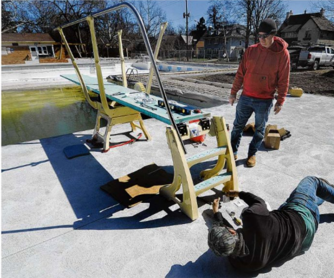
Shamrock Enterprises employees Ben Lykins (standing) and Tim Artrip install a new diving board stand at the Oakwood City Pool last month. MARSHALL GORBY / STAFF
