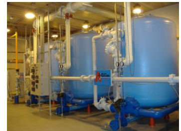
Softening Units at Shafor Water Treatment Plant
