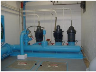
High Service Pumps at Springhouse
