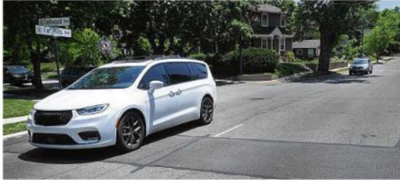
A $2.1 million sewer project is expected to slow traffic with lane closures for months on Far Hills Avenue from Dellwood Ave. to Greenmount Blvd. in Oakwood. MARSHALL GORBY / STAFF
