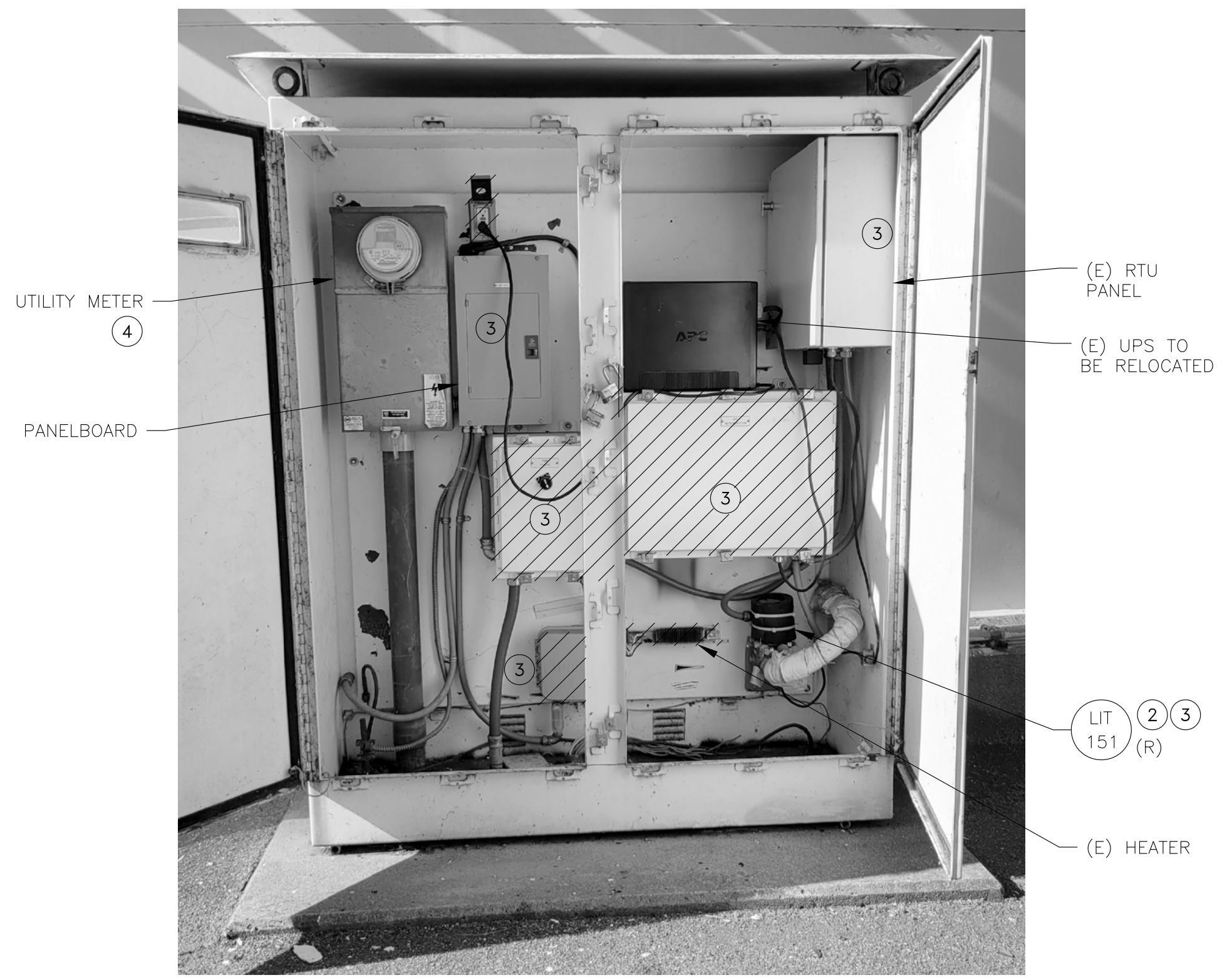
(E) ELECTRICAL CABINET (A) (E3) (1)
