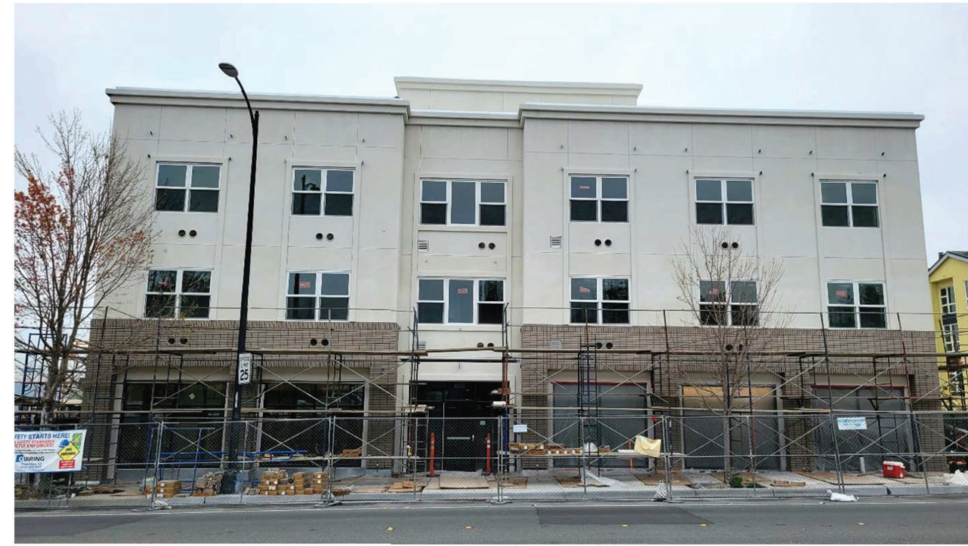
View from south of Project Site looking east at 4-story PBN 414 Apartments at 414 Petaluma Blvd. North.
