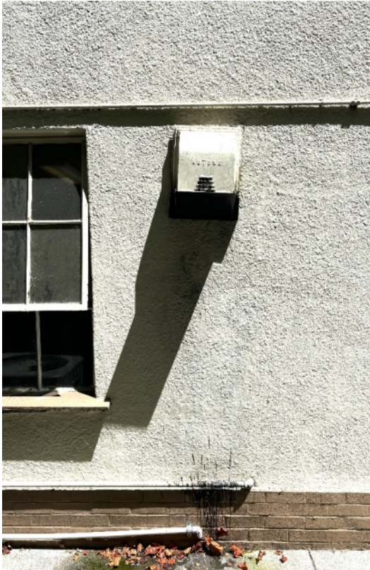
View of West elevation original 1938 kitchen exhaust hood with grease stains – Source: Report Author
