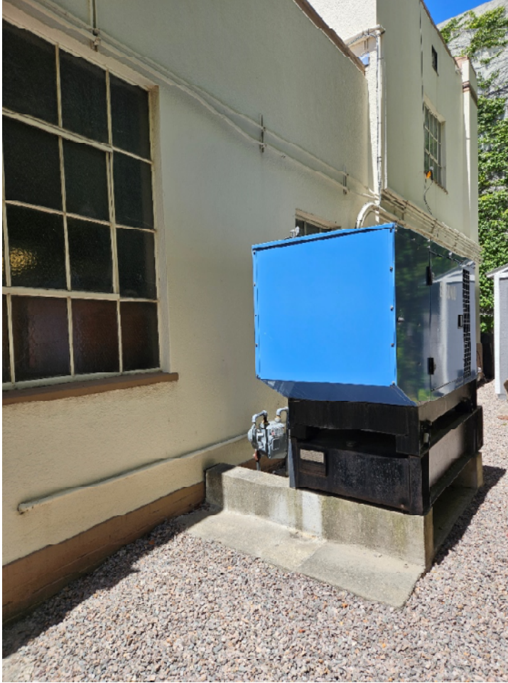
North side yard emergency generator. Air compressor to be located adjacent to generator Source: Report Author
