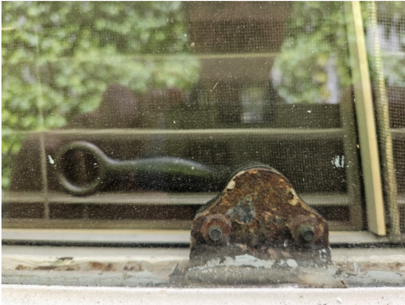
View of degraded window hardware – Source: Report Author
