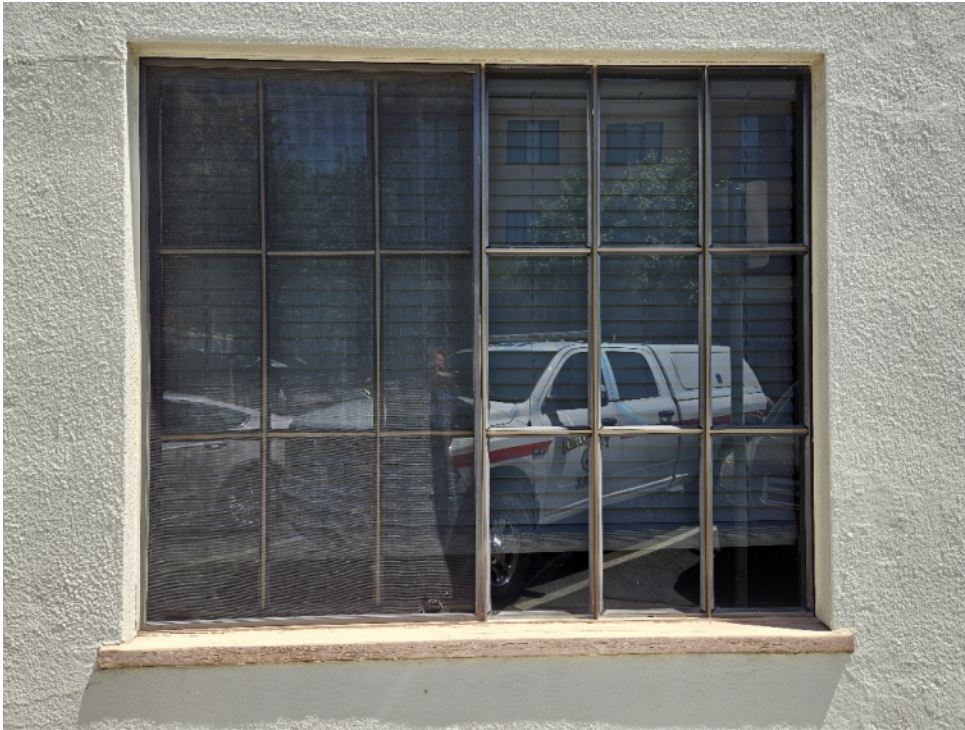
View of first floor South elevation 1970's aluminum window along Public Way – Source: Report Author
