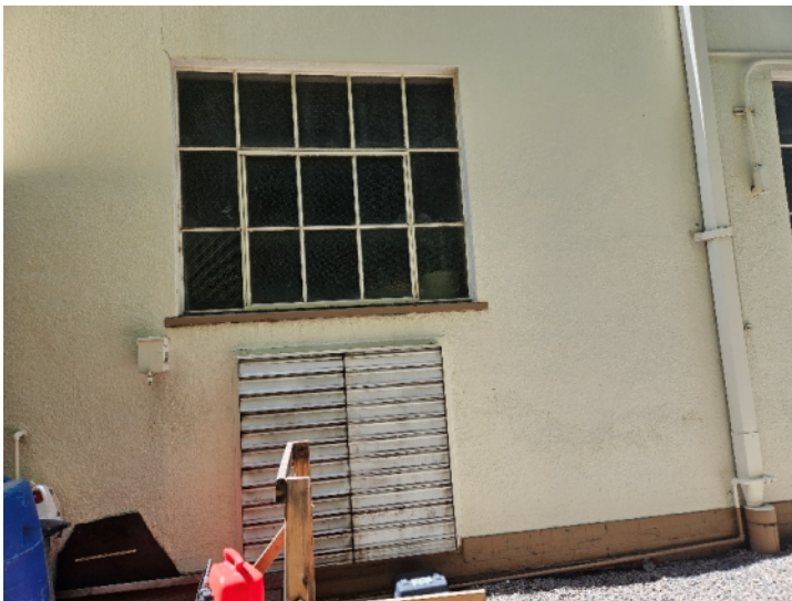
View of window and grille to be replaced with man door and grille – Source: Report Author
