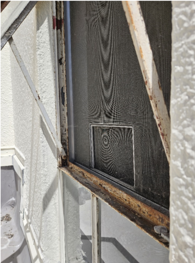
Exterior view of degraded South facing windows – Source: Report Author
