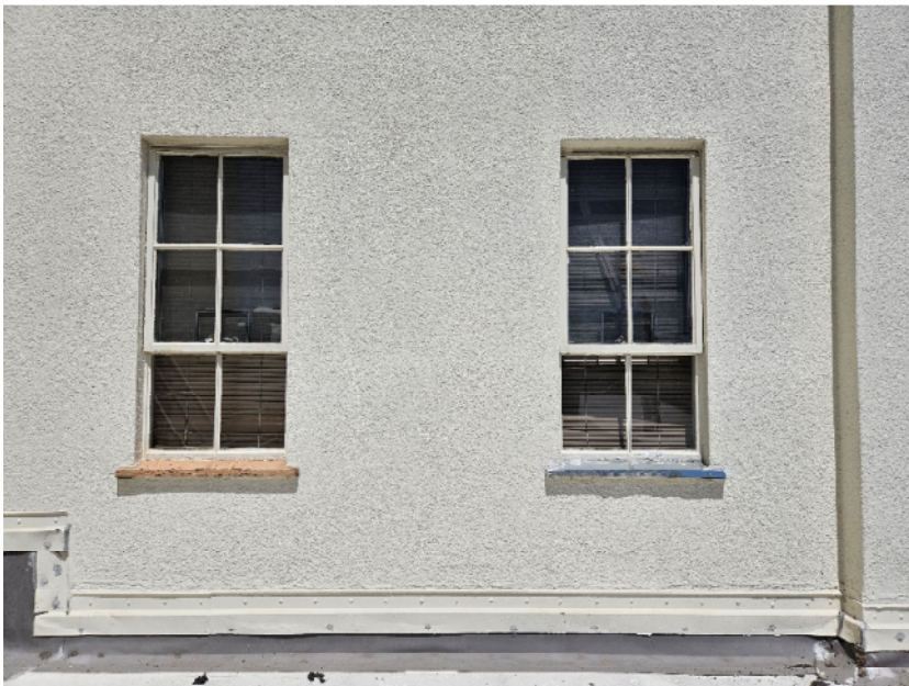
View of second floor East facing windows scheduled for replacement. Note degraded window sills Source: Report Author
