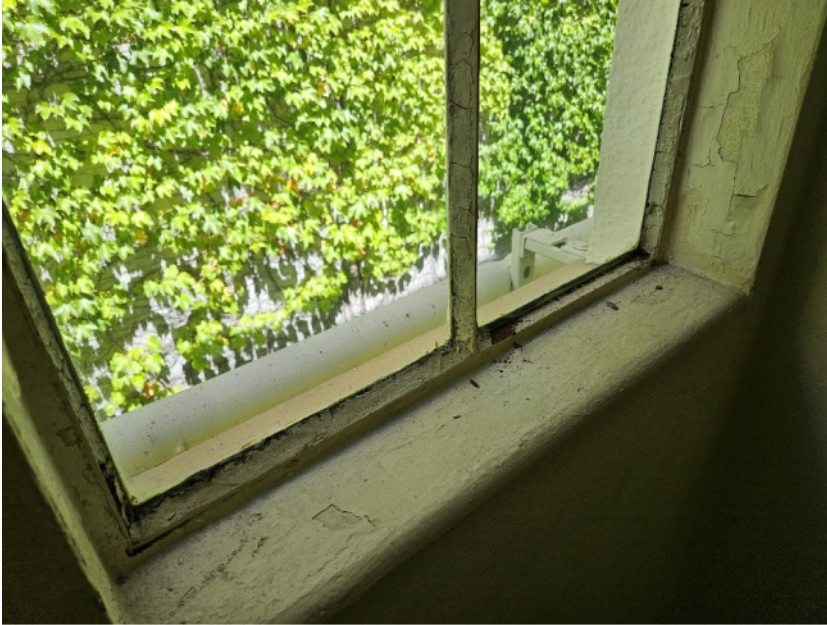
Interior view of degraded West facing windows – Source: Report Author
