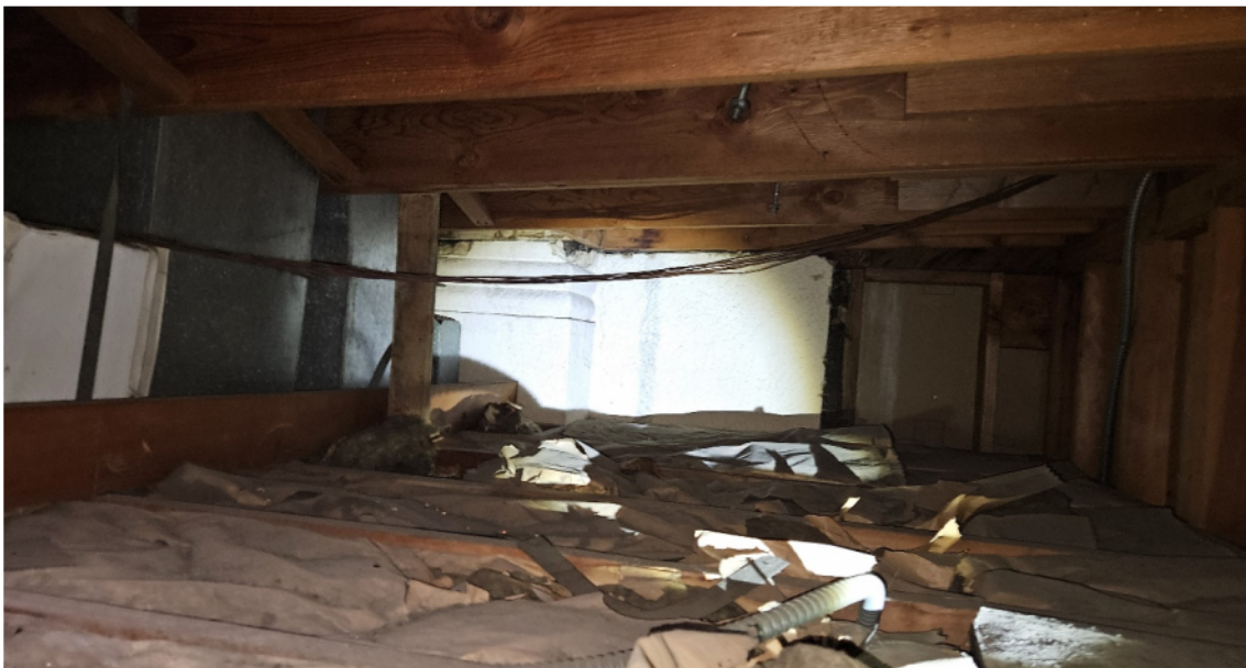
View of original 1938 construction from within ceiling plenum of 1970's addition. Source: Report Author
