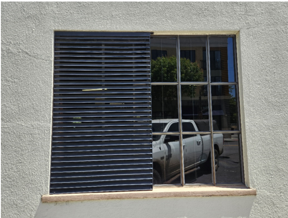
View of first floor South elevation 1970's aluminum window and steel exhaust grille – Source: Report Author
