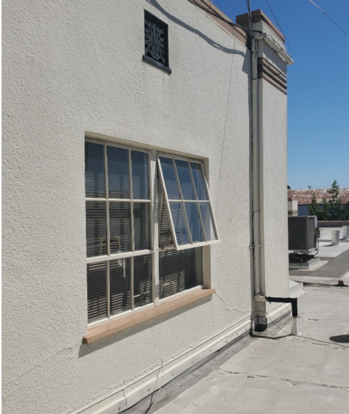
View of second floor South facing windows requiring replacement to meet exiting requirements Source: Report Author
