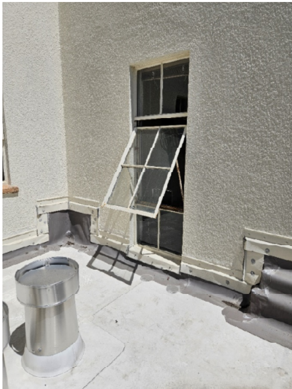
View of second floor South facing window requiring replacement to meet exiting requirements Source: Report Author
