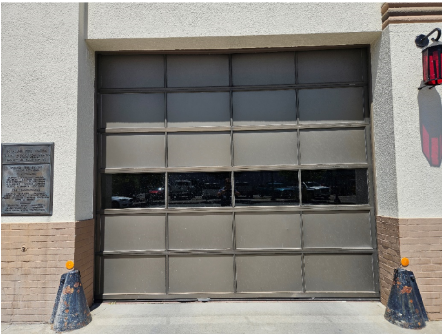
View of East elevation aluminum apparatus bay doors to be replaced – Source: Report Author
