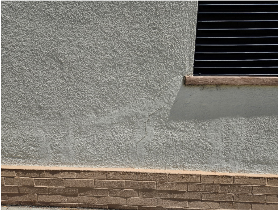
View of South elevation plaster cracks – Source: Report Author
