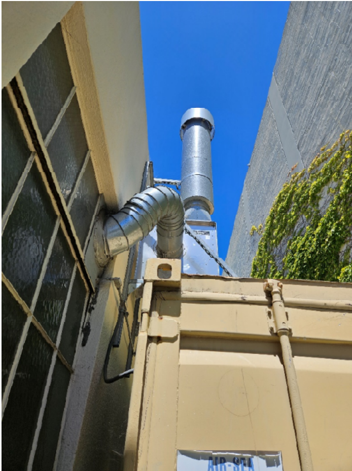
View of North Side Yard exhaust fan and ductwork as seen from the Public Way – Source: Report Author
