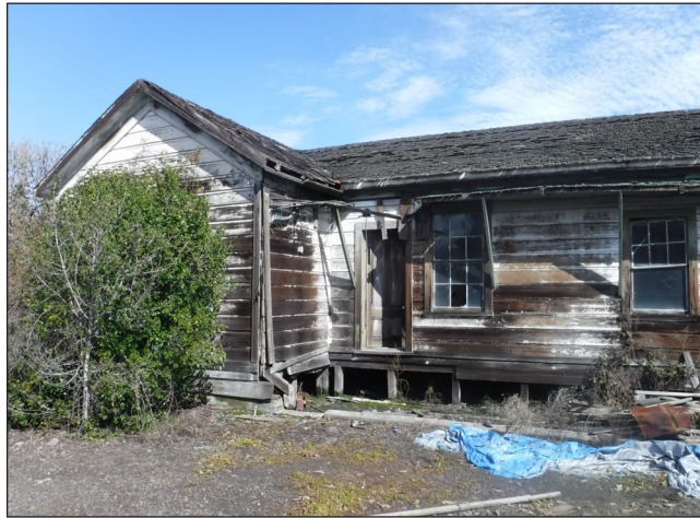
PHOTO 1: Abandoned house in disrepair on the southwest corner of the project site.
