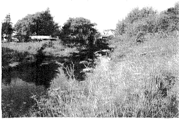
Flood protection for residences built very close to the river banks is recommended for the Payran Residential Segment .
