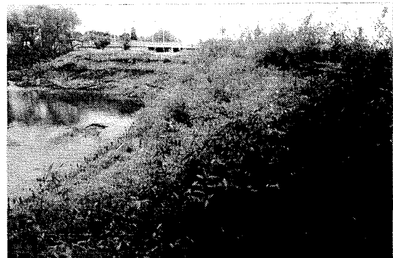
An example of a form of bio-engineering called willow wattling (a dense bundling and direct planting of willow cuttings) successfully protected this river bank at the Factory Outlet Mall during the 1994-95 storms.
