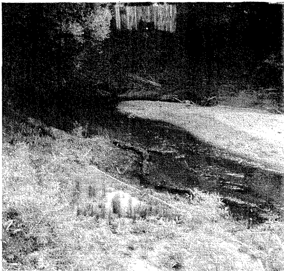
The left bank, near the Factory Outlet Mall, has been stabilized using a variety of bioengineering techniques, including willow wattling, seeded slopes, and coir matting at the toe.
