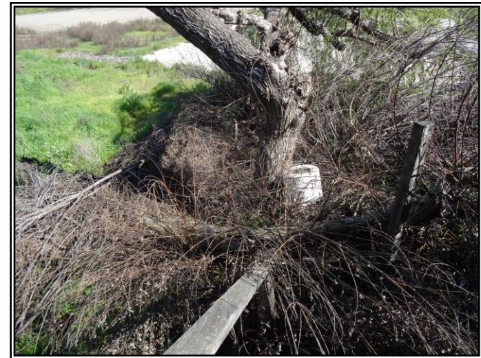
Looking at the tree limb obstructing the bottom portion of the stairs located to the east of Structure CC/DD.
