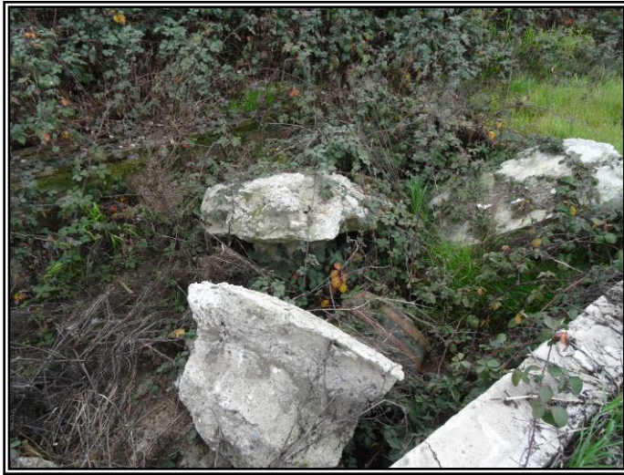
Looking at dumped concrete footing to the south of the concrete foundation.
