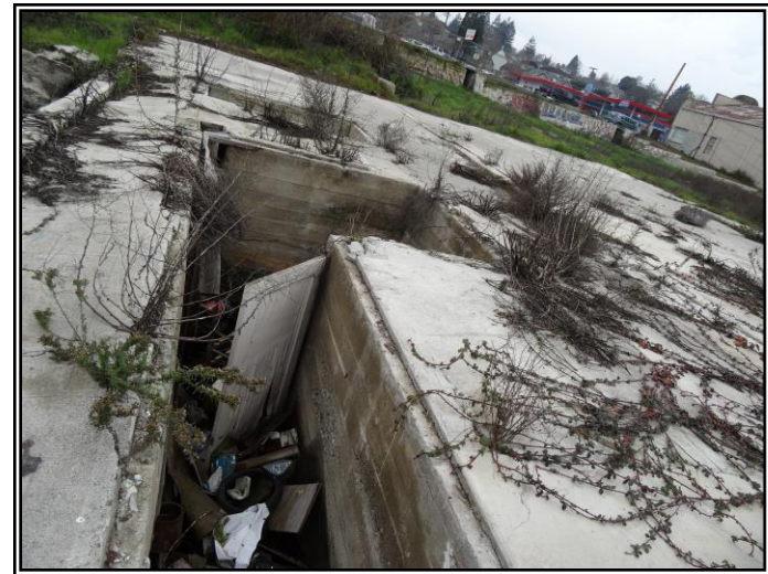
Looking at the access from the east to an opening in the concrete foundation.
