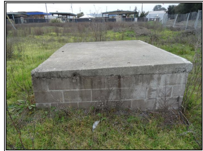
Looking at a concrete structure to the north of the fenced area.
