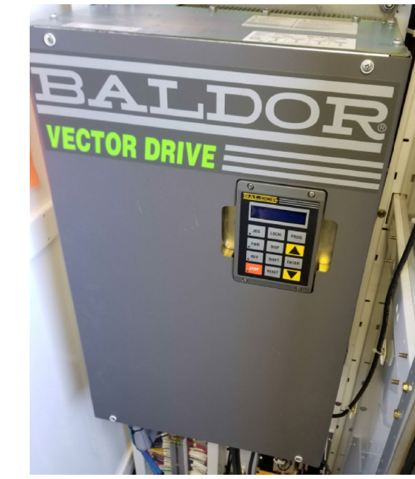
EXISTING VFD DRIVE
