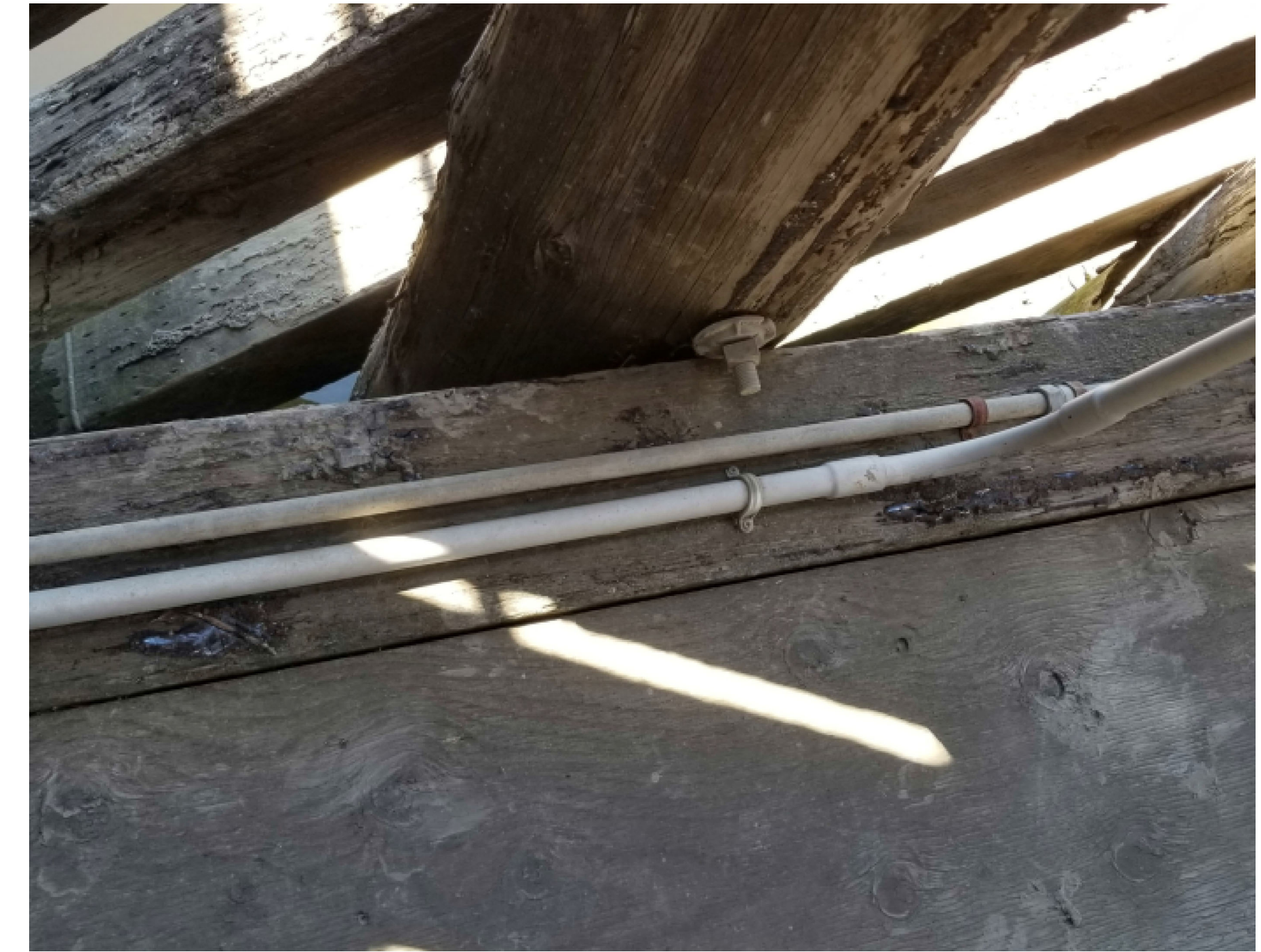
NAVIGATIONAL LIGHT CONDUITS RUNNING FROM WEST TO EAST ON THE SOUTH SIDE OF THE BRIDGE
