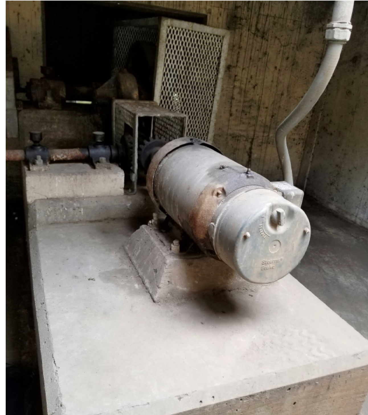
END LOCK MACHINERY MOTOR
