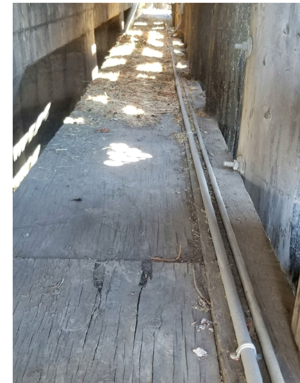
NAVIGATIONAL LIGHT CONDUIT AND CCTV CONDUIT RUNNING FROM WEST TO EAST ON THE NORTH SIDE OF THE BRIDGE
