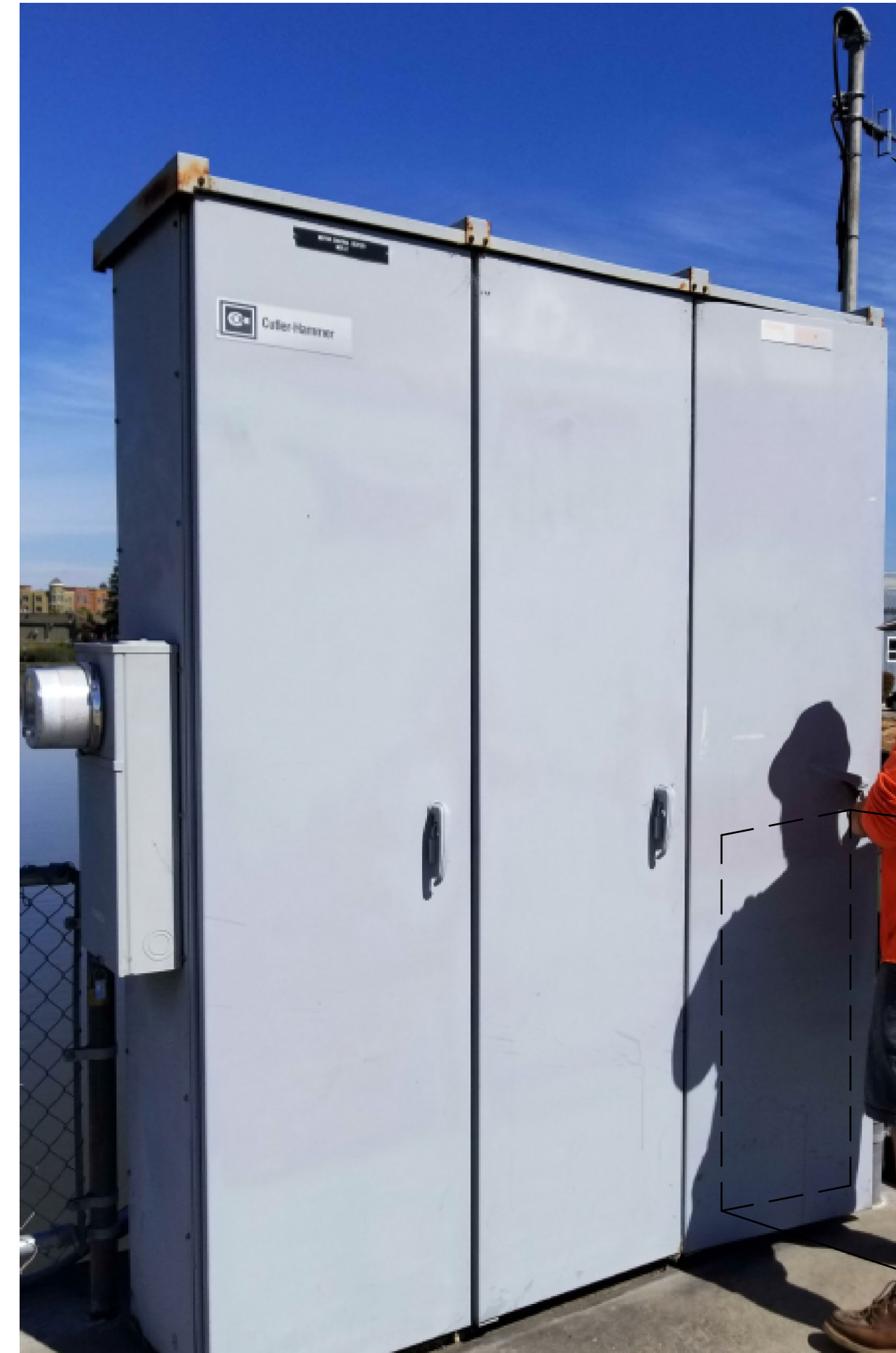
MCC-2 FRONT VIEW
