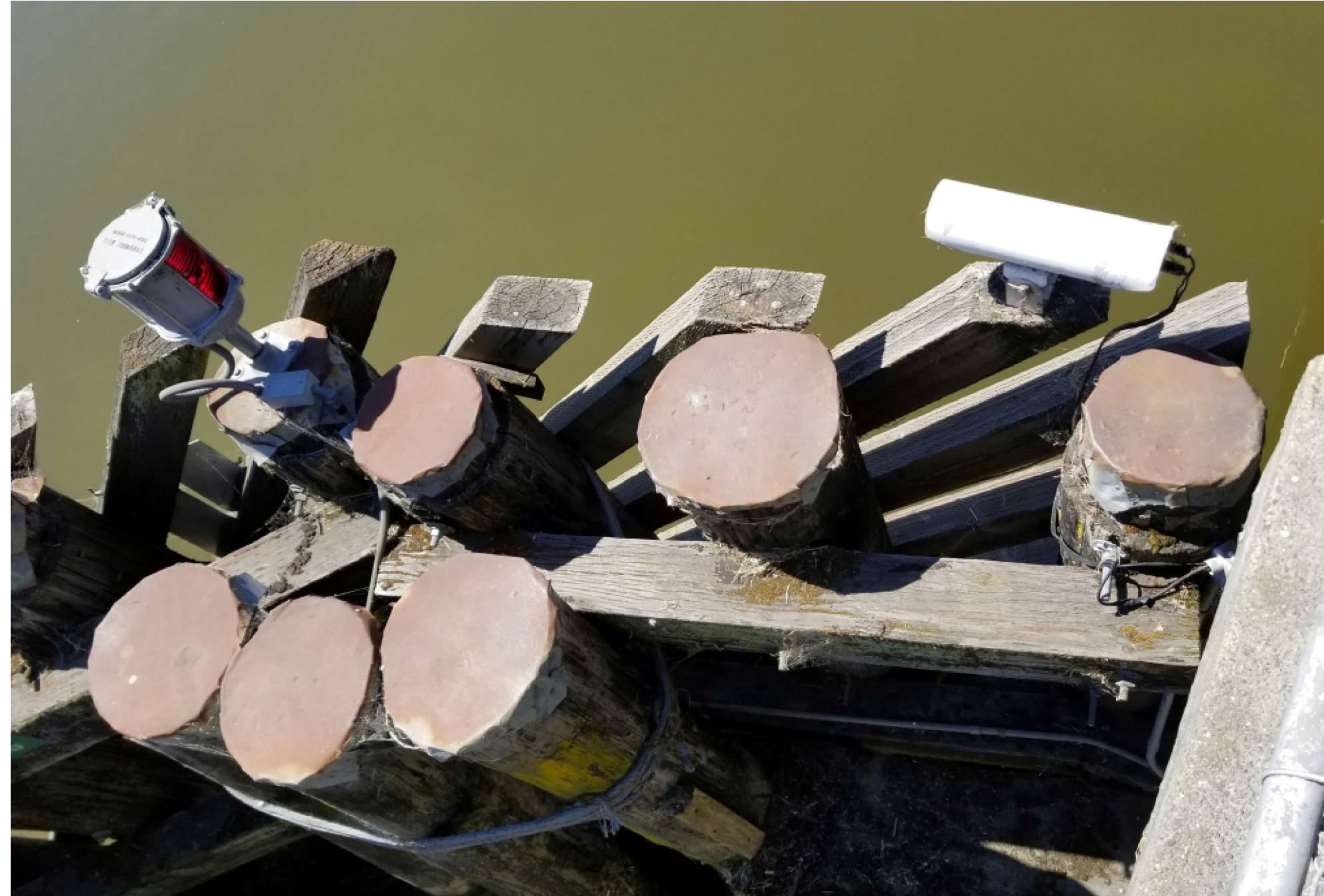
NAVIGATIONAL LIGHT AND CCTV CAMERA ON NORTH EAST SIDE OF THE BRIDGE
