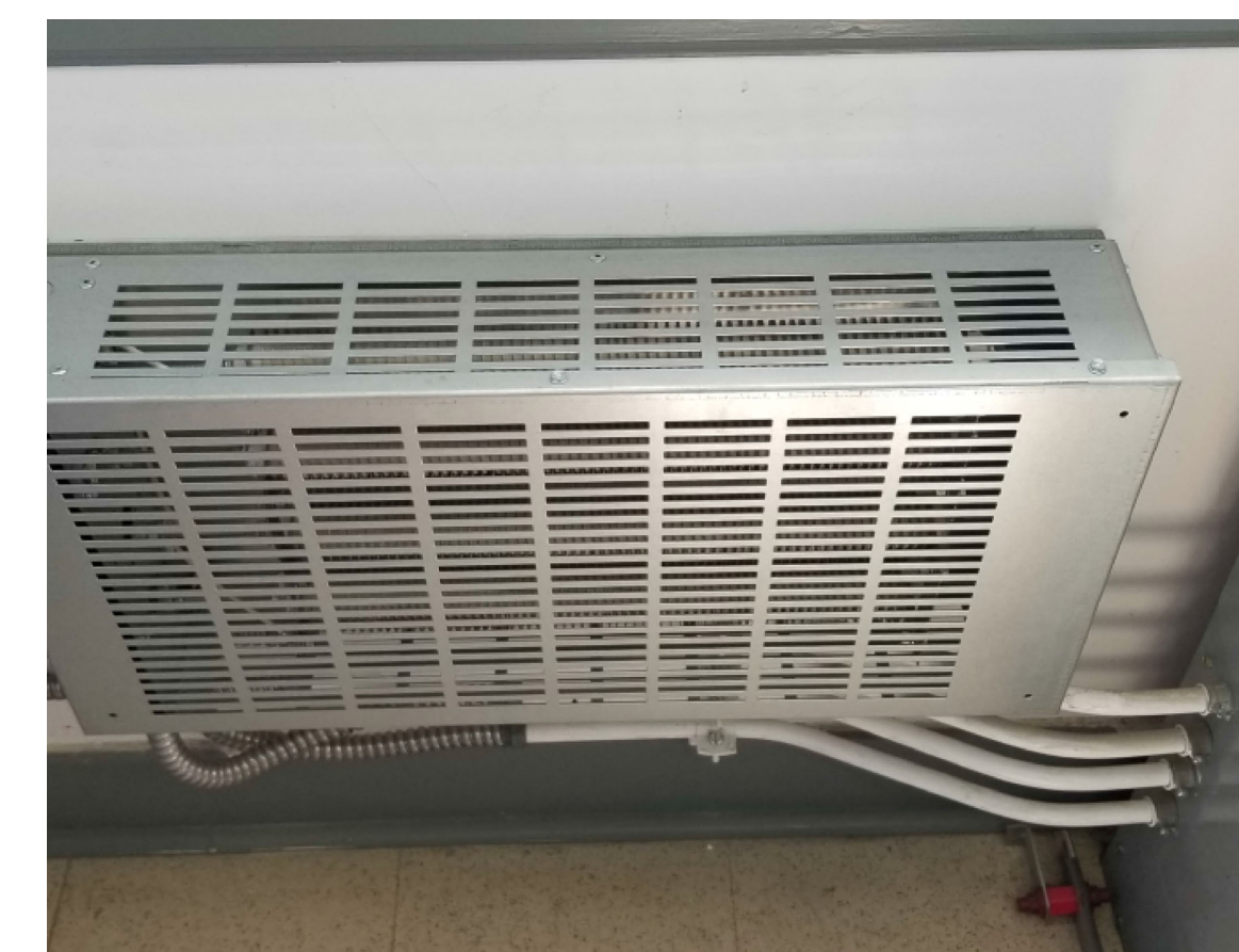
EXISTING BREAKING RESISTOR
