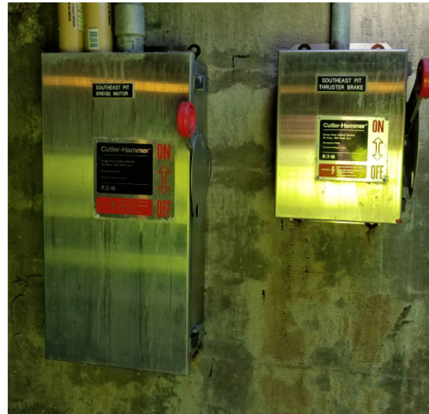
NORTH WEST THRUSTER AND MAIN MOTOR DISCONNECTS
