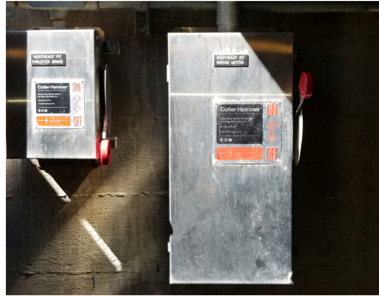
NORTH EAST THRUSTER AND MAIN MOTOR DISCONNECTS
