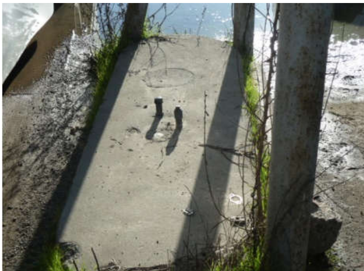
Photo #24: Plumbing within pump island
