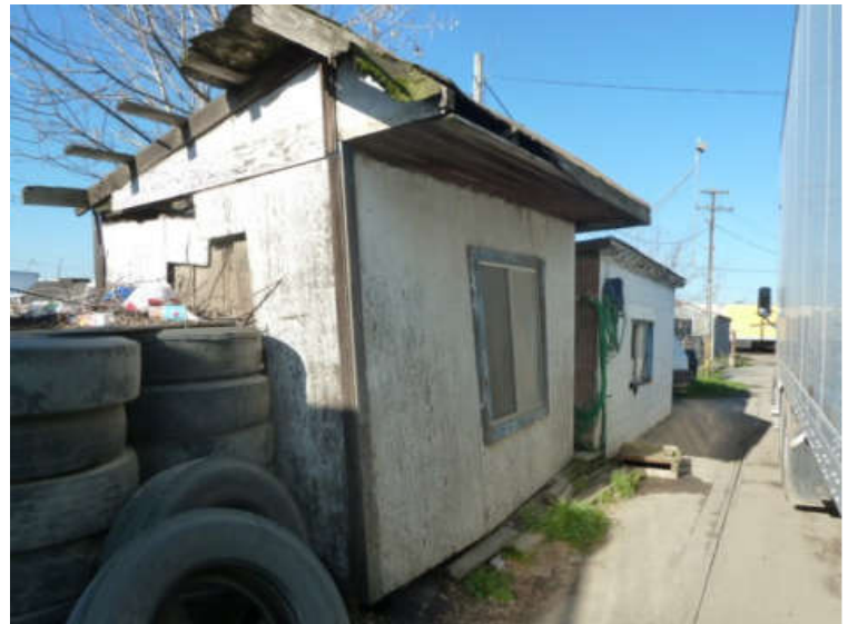
Photo #26: Truck scale house (masonry, right) and wooden shed (left), both locked during visit
