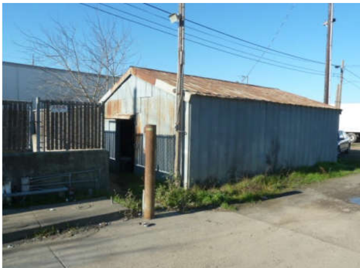
Photo #21: Well house shed (right) and former AST storage areas (left); noted former dispenser piping in front of AST concrete berm
