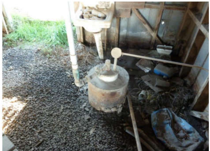
Photo #20: Groundwater well within well house shed
