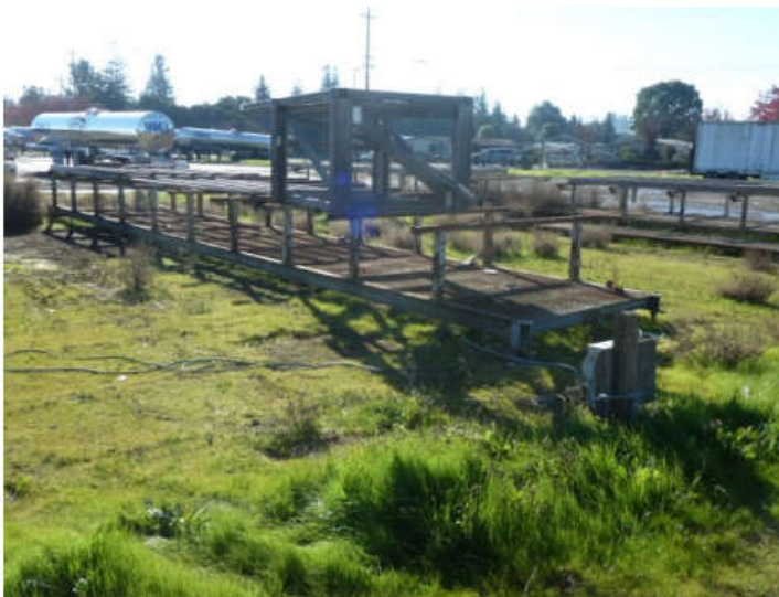
Photo #36: Truss assembly area. One of 6 stations, each with electrical and compressor plumbing (front left)
