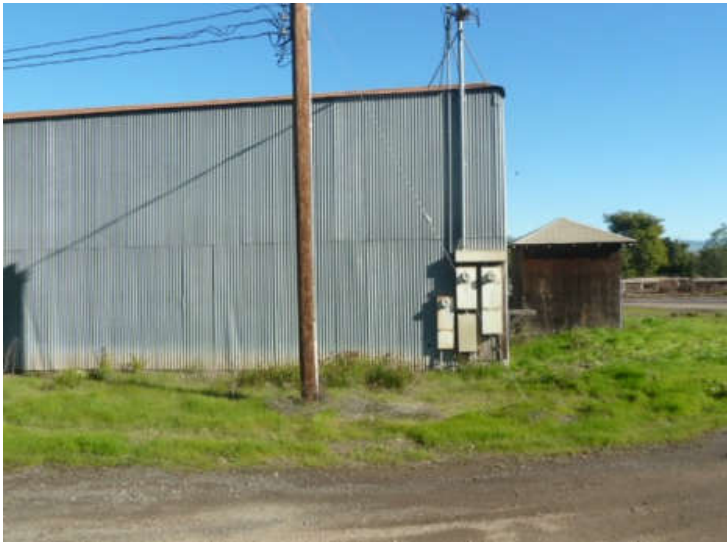
Photo #37: Electrical on southeast corner of central metal building, compressor shed (right)
