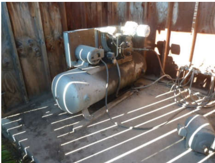
Photo #33: Compressor shed on east side of central metal building
